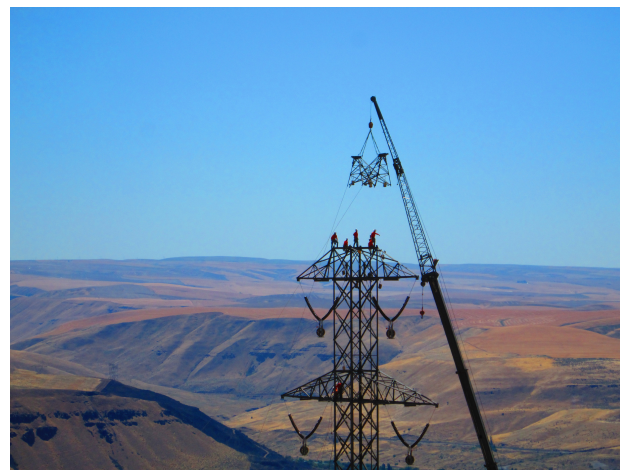
Major upgrades to the country's transmission lines are included in infrastructure legislation.
